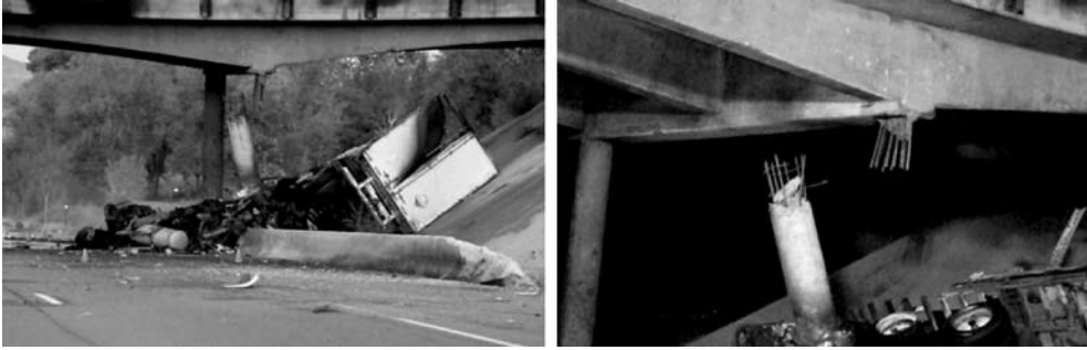
Fig. 7. The Road 26.5 bridge in Grand Junction (Colorado, US) lost a support column and was closed after it was hit by a semi-truck on August 15, 2007
