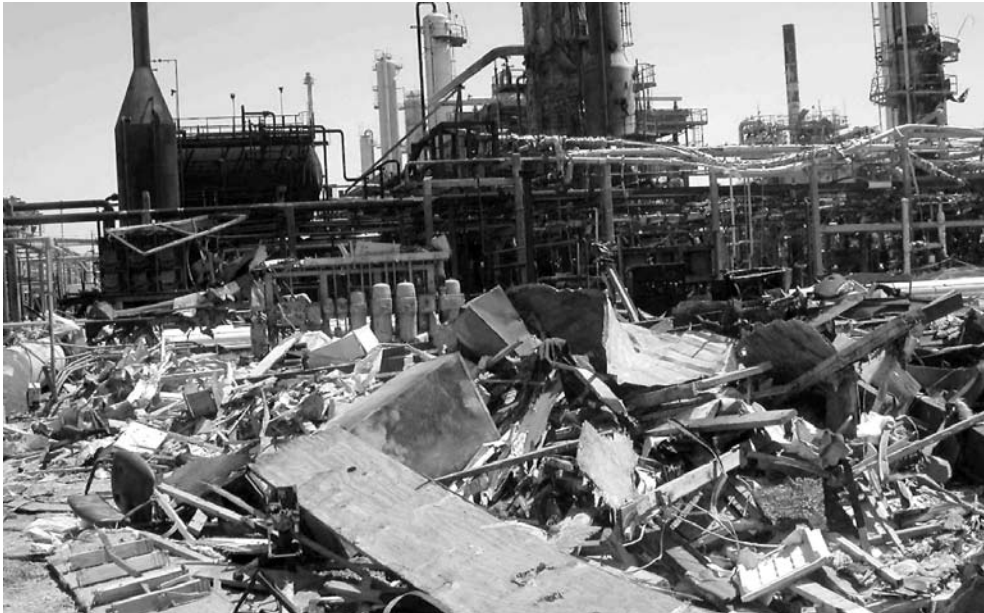
Fig. 3. Explosive damage to technological piping (top-right side of the picture; BP Texas City explosion March 2005) (CSHIB 2005)
