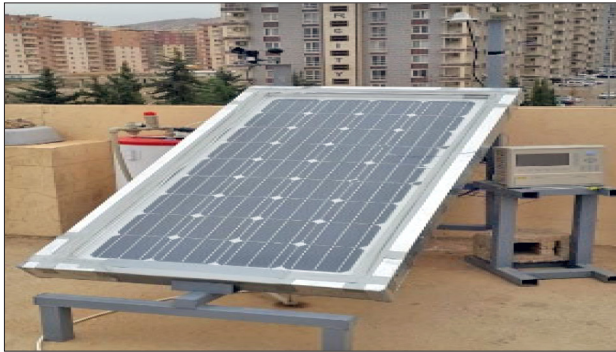
Figure 2. Front view of the PV/T collector
