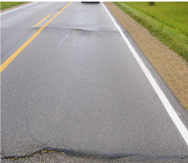
Fig. 9. Picture of reflection cracking on AC-overlaid virgin PCC pavement (No. 6: IA139 in Winneshiek County)
