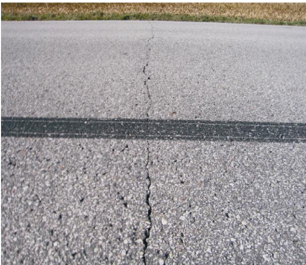
Fig. 8. Picture of low-temperature cracking on AC-overlaid rubblized PCC pavement (No. 3: D16 in Black Hawk County)
