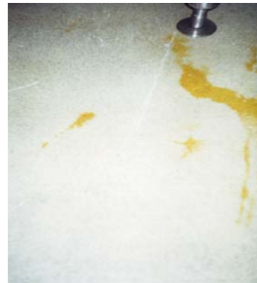
Fig. 3. PERAN system coating coloured due to constantly running water from the system, JSC Rokiškio sūriai
