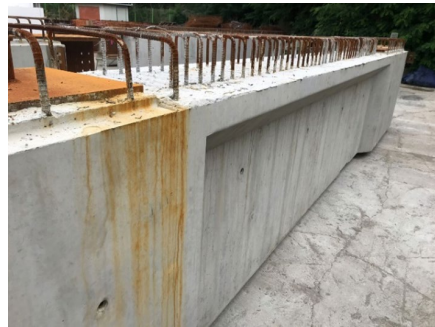
Figure 12. Repair case: chemical treatment was applied to repair discoloration on the PC beam surface stored in a storage yard due to the corrosion of exposed bars
