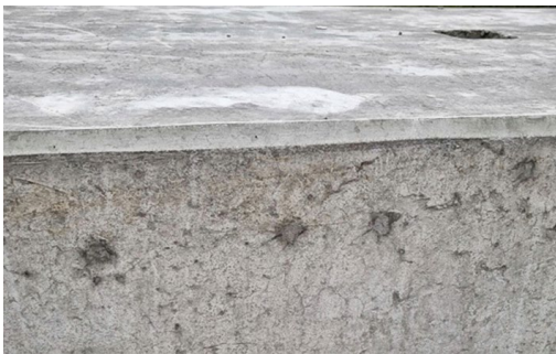
Figure 11. Repair case: small holes on the side of a PC wall component filled with mortar
