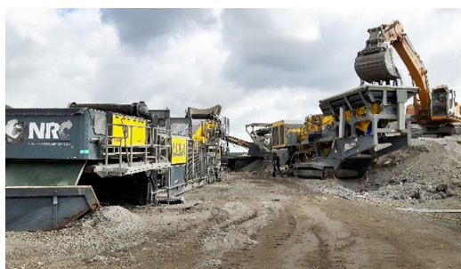
Bottom ash is supplied to metals recovery system
